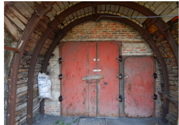
Figure 6. Image of a manually operated ventilation gate with a brick wall and iron frame at the +30 tunnel in the Canh Dong area of Mong Duong Coal Mine
